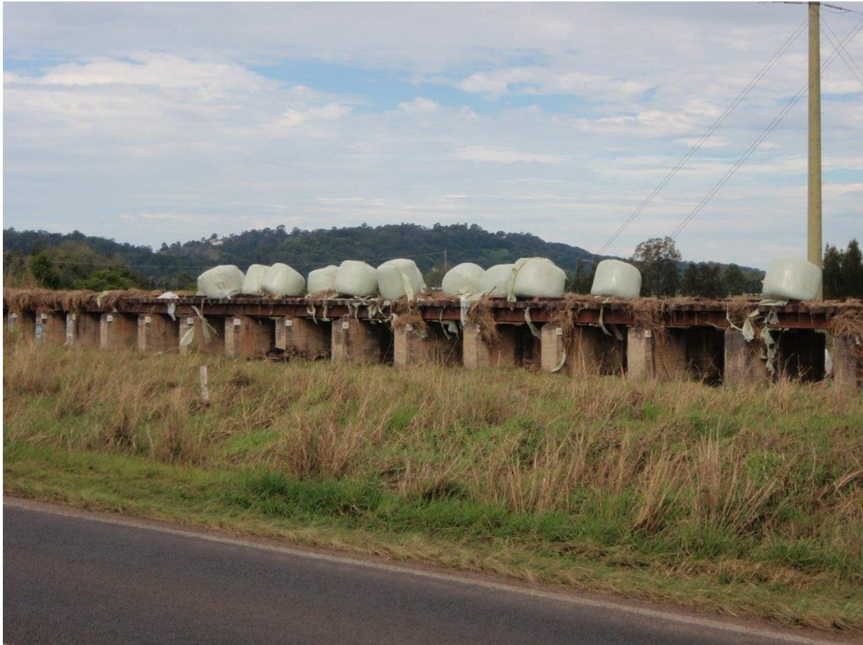
Leycester Creek, Tuncester 23 May 2017, hay bales lifted by the flood onto the railway tracks
